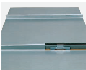
Fig. 3: Installation of a sealing strip to the undercloak that has been fastened with clips.
